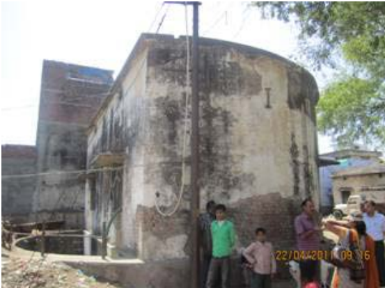
Site for SPS-Mahigram (existing SPS will be demolished and a new one will be constructed)
